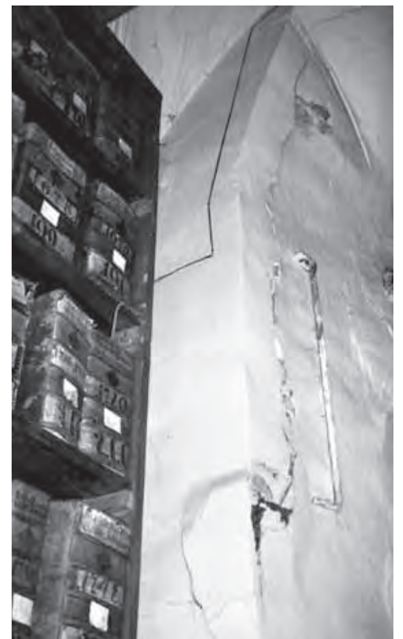
A cracked interior wall in former Bernardine monastery, which houses the Central Historical Archives.
