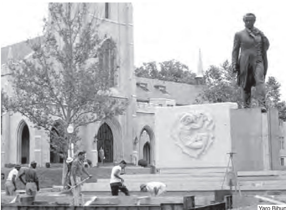
A construction crew — all Black Americans — hurries to complete the Shevchenko monument grounds in time for its dedication ceremony to take place June 27, 1964 — one week before President Lyndon Johnson would sign the landmark Civil Rights Act outlawing racial segregation in the United States. It would be another year until the Voting Rights Act outlawed all discriminatory voting practices used against Black Americans in the United States.
