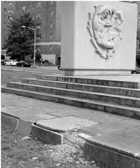
The cracked and missing concrete pavers just to the left of the Shevchenko Memorial one hour before the Washington Ukrainian community came to honor his birthday in 2012.
